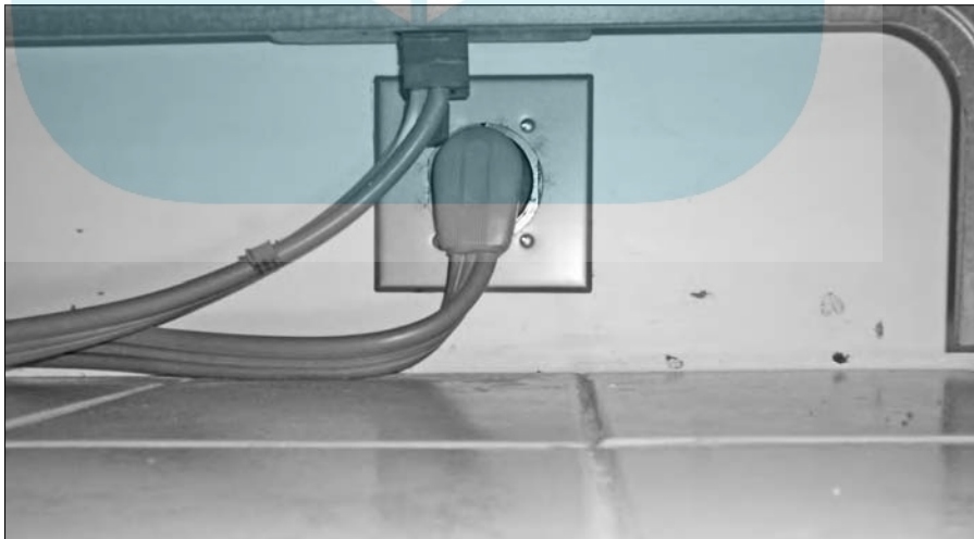
Figure 3-13: A typical 240-volt receptacle for an electric range.
